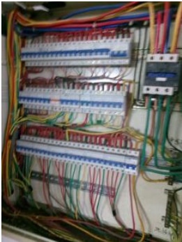
Electrical control panel without inner cover.JPG
